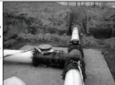
A single main pipeline reduced diversion and increased streamflow during critical flow periods.
