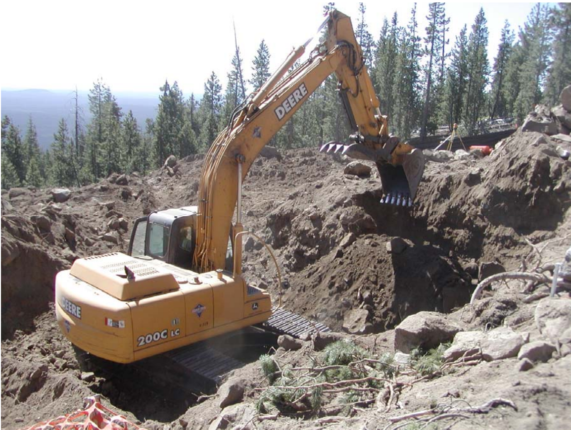
Photo courtesy of Bonneville Power Administration.
