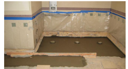
Above - Cedar Unit shower room concrete pour. Concrete substrate is ready for a mortar bed that will be topped with ceramic floor tile.
