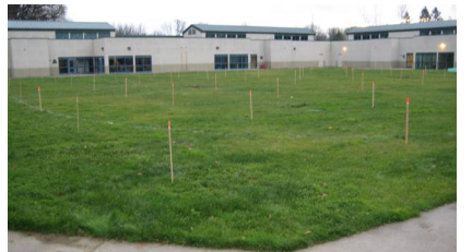
Above - Central courtyard grid layout; for positioning the location of side walks, the reflective pond, trees and furnishings.
