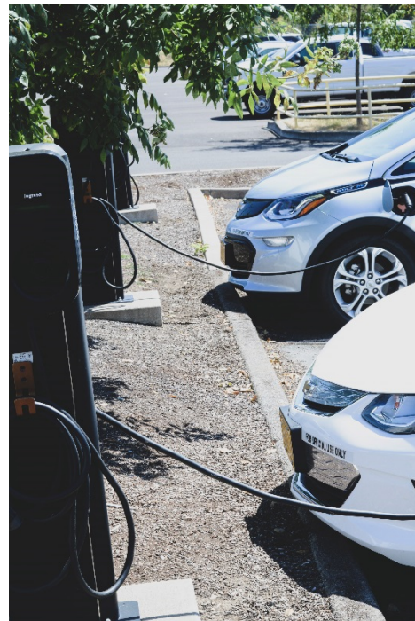
EV charging at Salem Motor Pool
