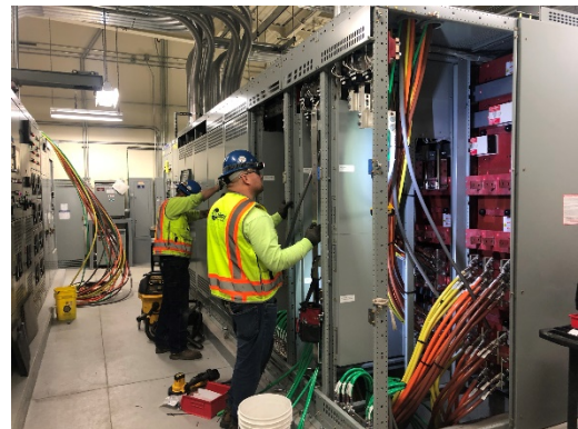
Energy efficiency upgrades at the State Data Center.
