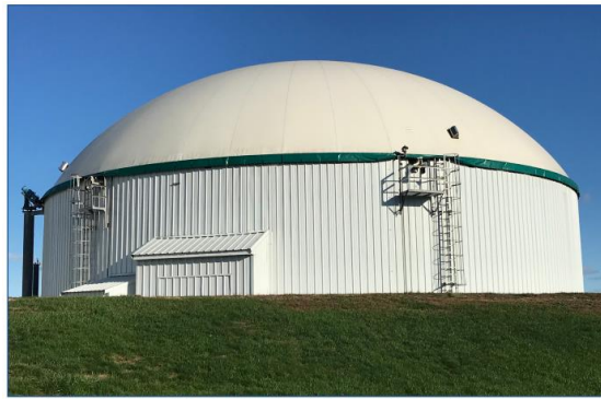
Photo 1: Dairy Biogas Anaerobic Digester Facility, Clean Fuel Partners, LLC, Dane, WI
