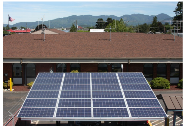
Tillamook PUD's headquarters has solar on site.
