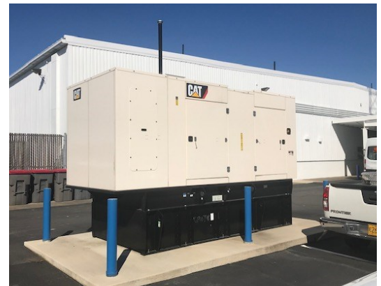
McMinnville's generator will help keep operations running after an emergency.
