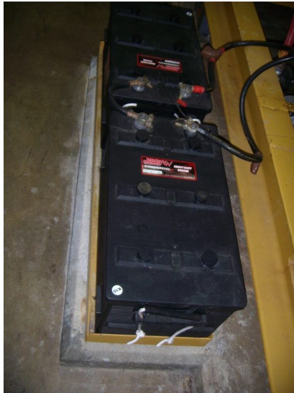
Figure 22. Batteries for the emergency generator at the City of Lincoln City Water Treatment Plant. The batteries have not been seismically restrained and may not operate the generator after a Cascadia earthquake.
