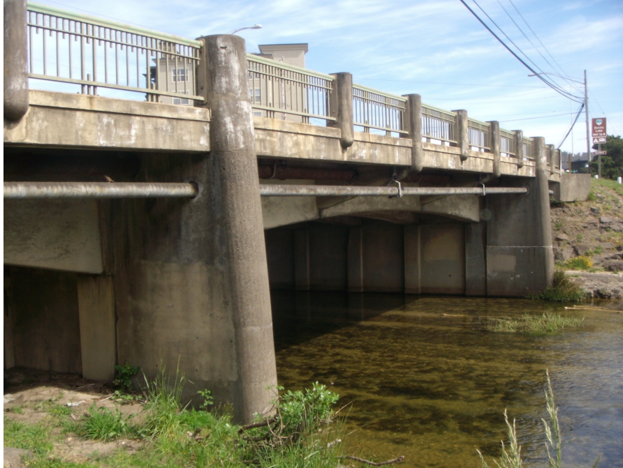
Figure 33. A 10-inch-diameter water transmission pipeline is colocated on the D River bridge on coastal Highway 101. This bridge is expected to experience tsunami inundation; in that event the pipeline is expected to incur breaks caused by bridge damage. A new, more reliable transmission pipe will be constructed under the river.
