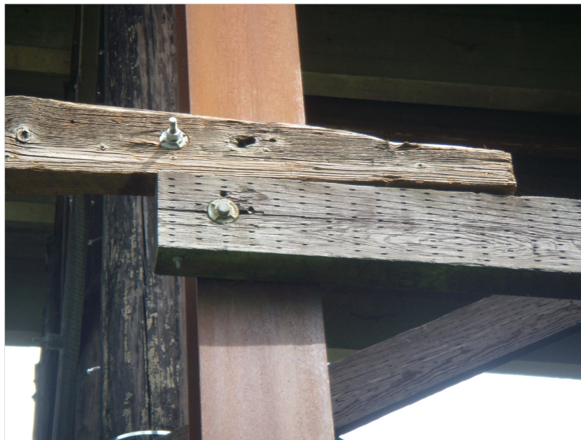
Figure 31. Close-up of Three Mile Lane bridge showing various ages and types of materials in the substructure, including steel and wood. This photo shows the inadequate seismic design, construction and maintenance, including split timber members. As supported by our analyses, it will likely be inoperable after a major earthquake.
