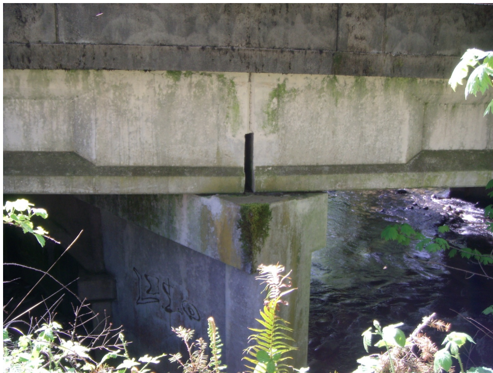
Figure 29. Bear Creek bridge on Highway 18 is expected to incur major damage during a Cascadia earthquake (Nako and others, 2009). One seismic deficiency relates to the inadequate width of the bearing seats; the bridge deck girders could slip off their supports during horizontal ground motions and render the bridge inoperable.
