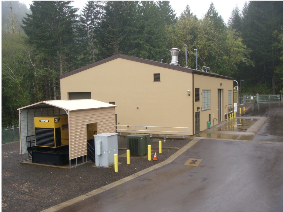
Figure 24. McMinnville Water and Light Water Treatment Plant showing the chemical building and emergency generator (foreground).
