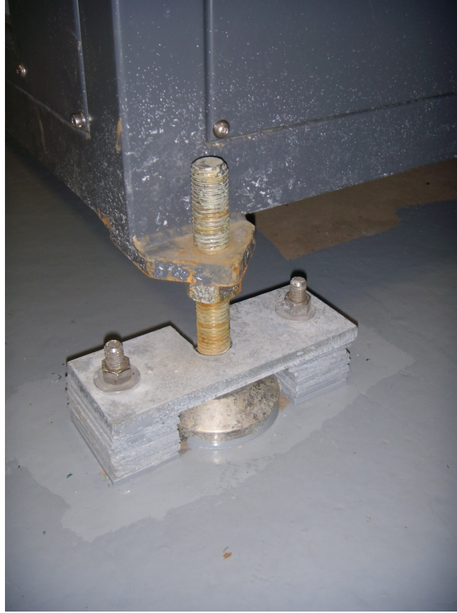
Figure 25. McMinnville Water and Light Water Treatment Plant showing equipment without adequate seismic anchorage. Note the missing upper nut on center bolt. Proper seismic restraints of mechanical equipment may require seismic analyses.
