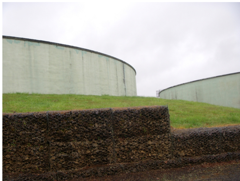
Figure 27. McMinnville Water and Light showing two of the four Fox Ridge Reservoirs. These are the pre-stressed concrete tanks.
