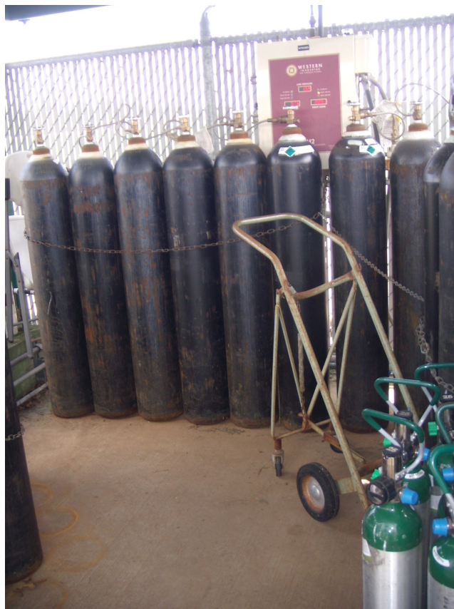
Figure 20. Medical gasses at McMinnville hospital (Willamette Valley Medical Center) are stored without seismic considerations.
