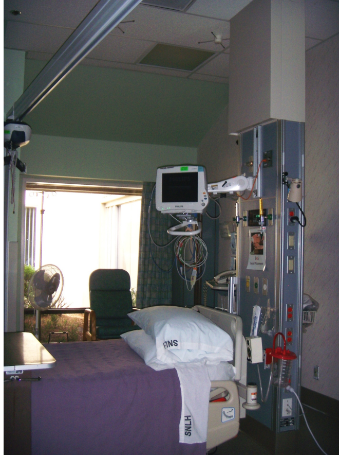
Figure 16. Lincoln City (Samaritan North Lincoln) hospital patient room with nonstructural damage potential, such as falling suspended ceiling tiles and medical equipment.
