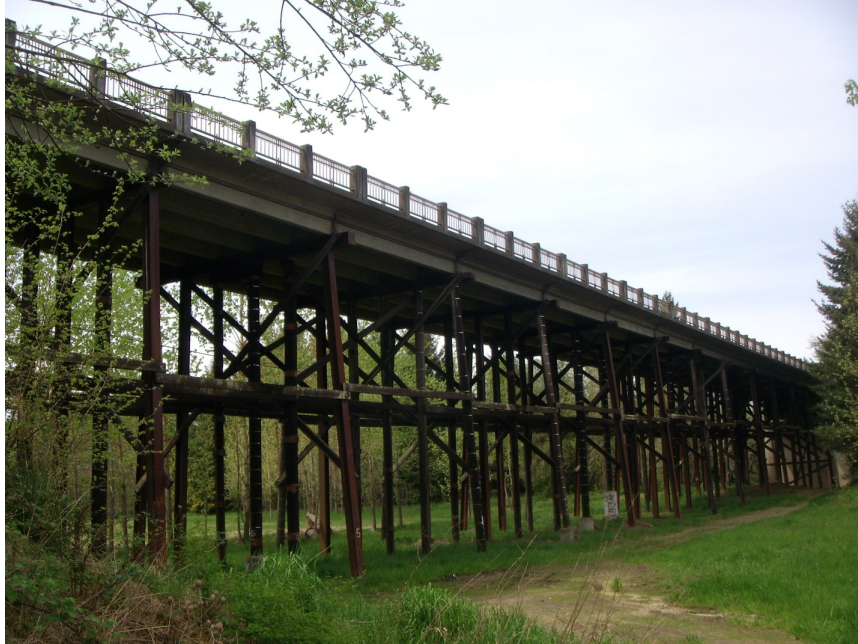
Figure 30. The 1951 Three Mile Lane bridge crosses the Yamhill River and connects downtown McMinnville and the hospital. It is in poor condition and has a telecommunication main line colocated on it. See Figure 30 and Figure 31.
