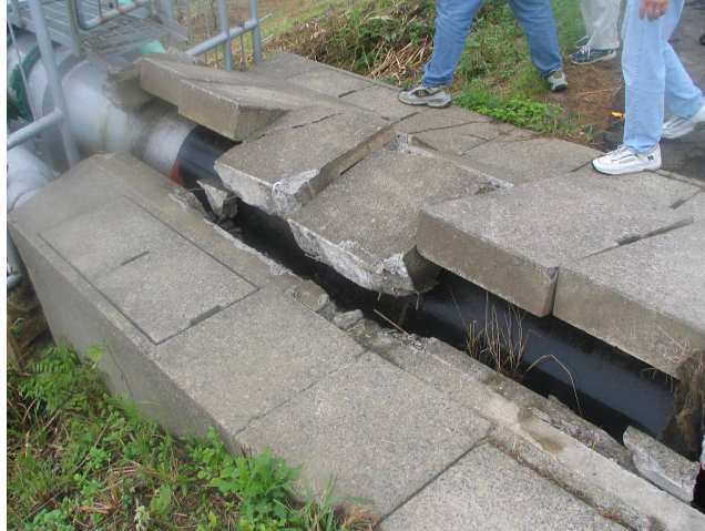
Figure 6. Water transmission pipeline failure at a river crossing in the 2007 Kashiwazaki, Japan earthquake.
