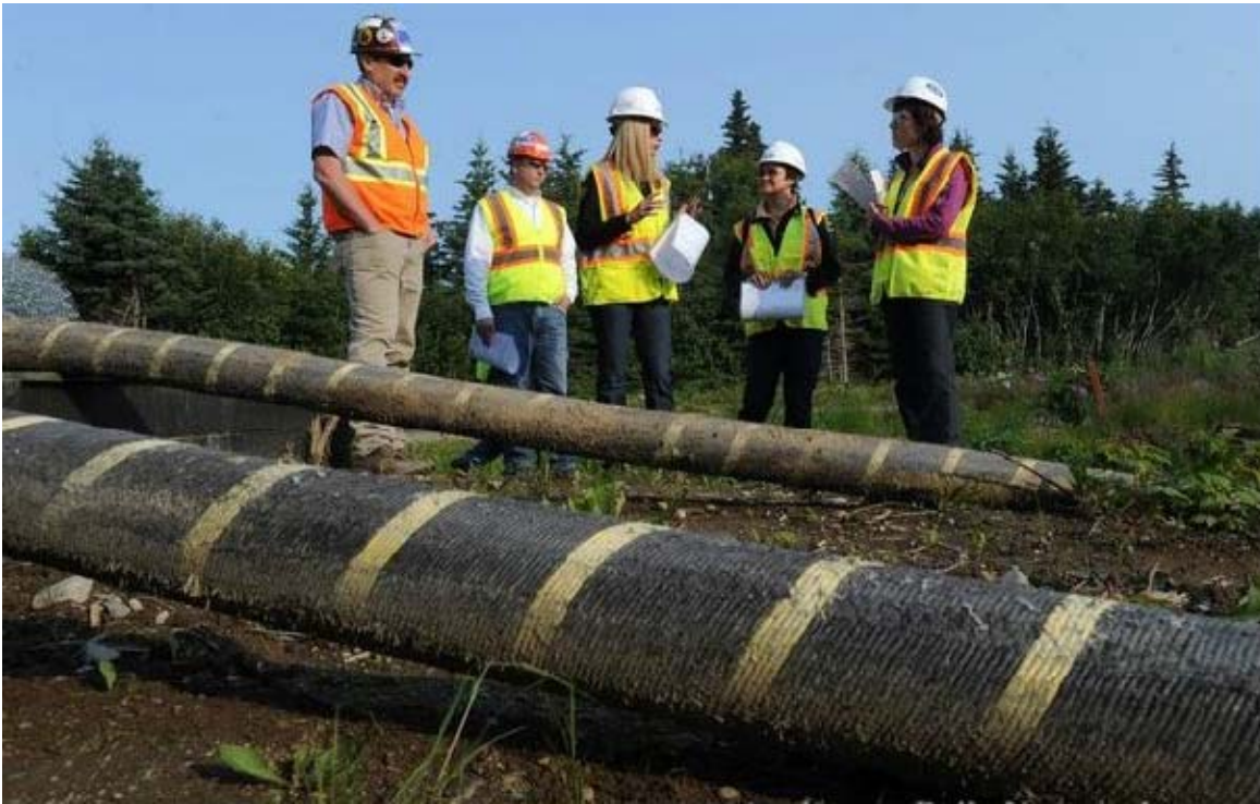
Deployment of submarine power cables, deployed for Fire Island Wind Farm in Alaska, 2012. Credit: Bill Roth / Alaska Dispatch News.
