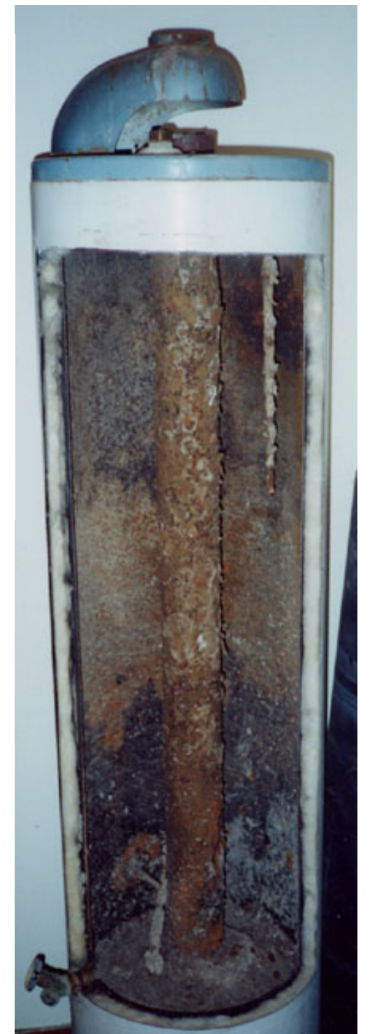
Water Heater Scale
