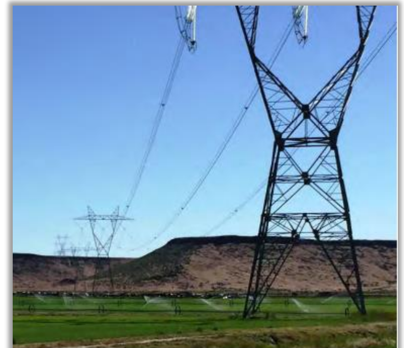
500-kilovolt (kV) transmission line near Melba, Idaho
