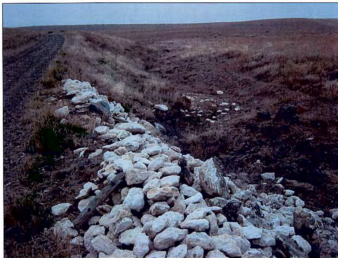
Photo Plate 14 View west showing stream channel adjacent to roadway at S12. White rock in foreground is a revetment for an apparent bank failure at this location.
