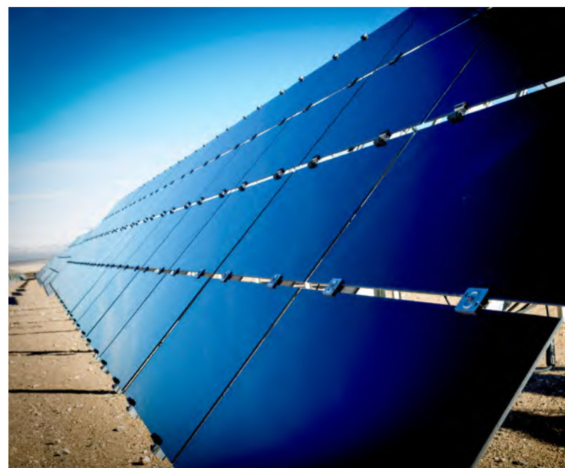
The 250-megawatt Silver State South Solar Energy Center in Nevada.
