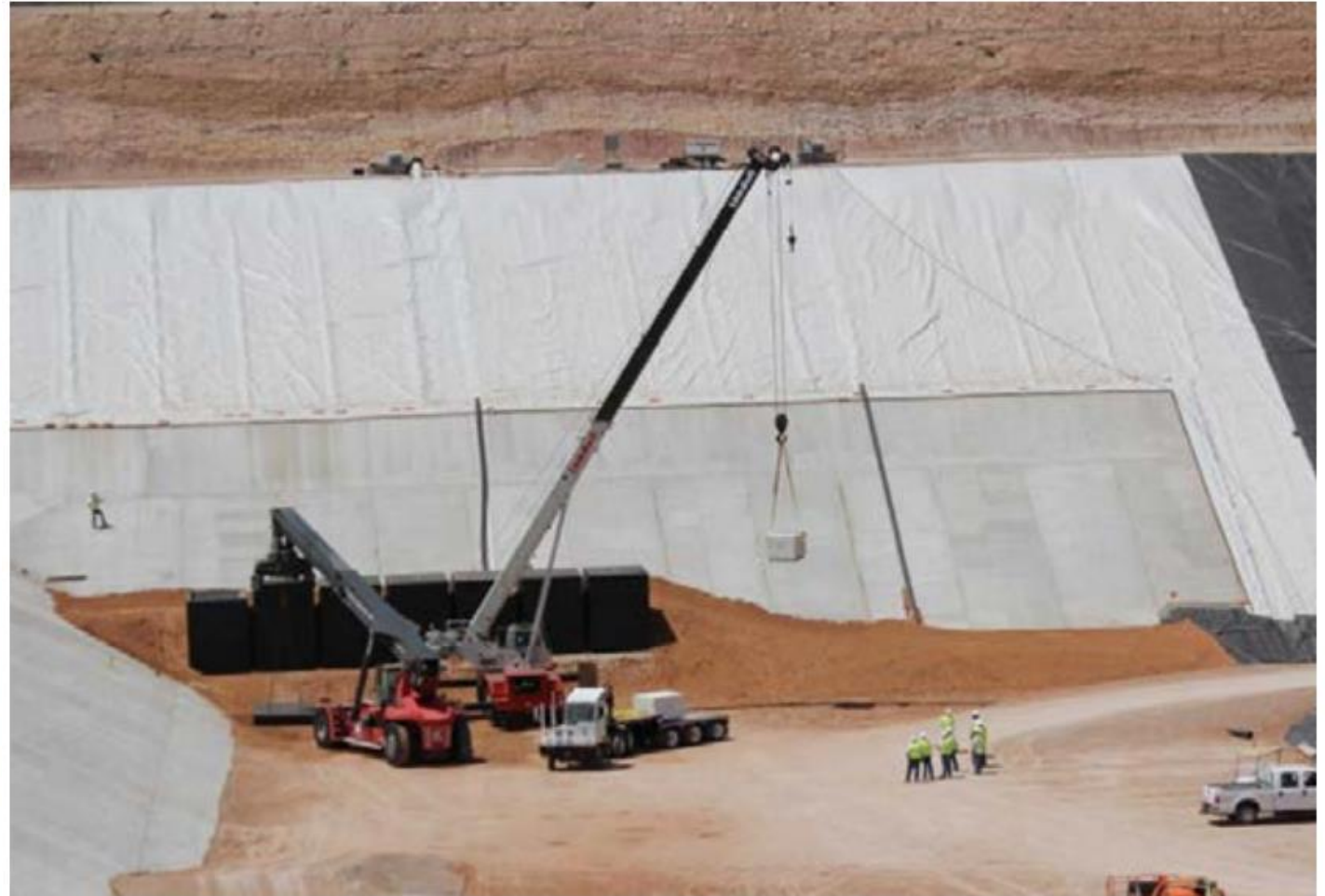
Figure 5-2 A Waste Control Specialists Disposal Cell and Wastes Being Placed in Modular Concrete Canisters (note workers for scale)
