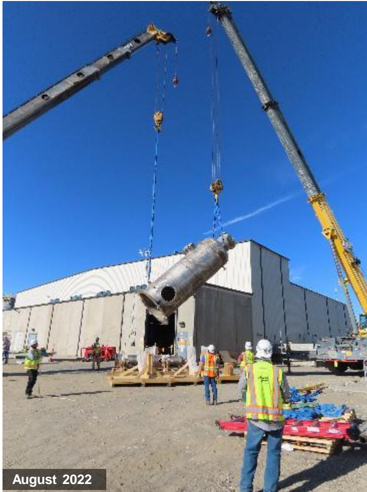
New Effluent Treatment Facility steam stripper
