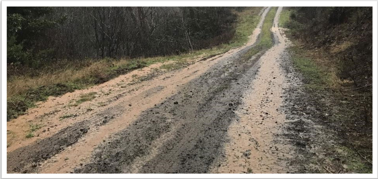
Photo 6. Rutted road, road shape does not move water off the road surface.
