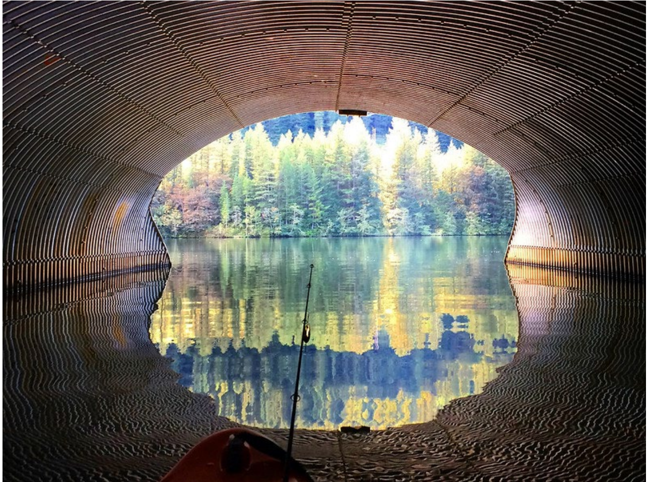
Culvert connecting North Fork Clackamas River to North Fork Reservoir, Linn, Oregon
