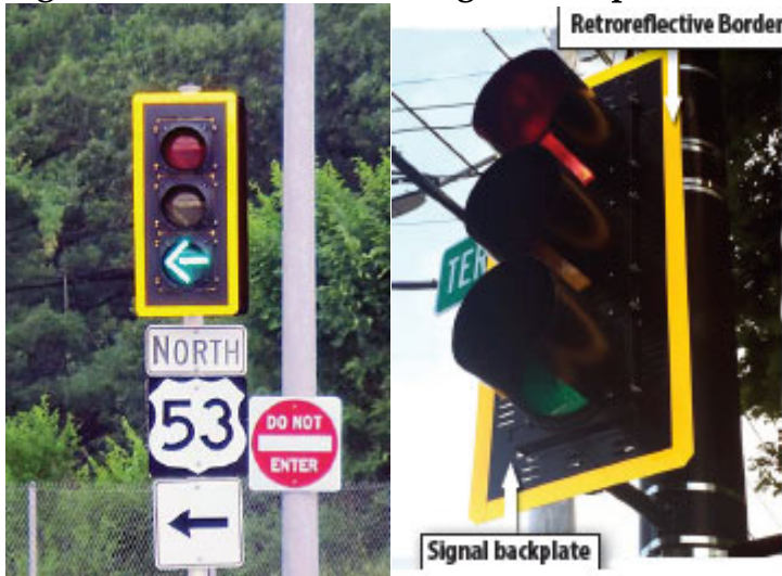
Figure 4-3. Retroreflective Signal Backplate
