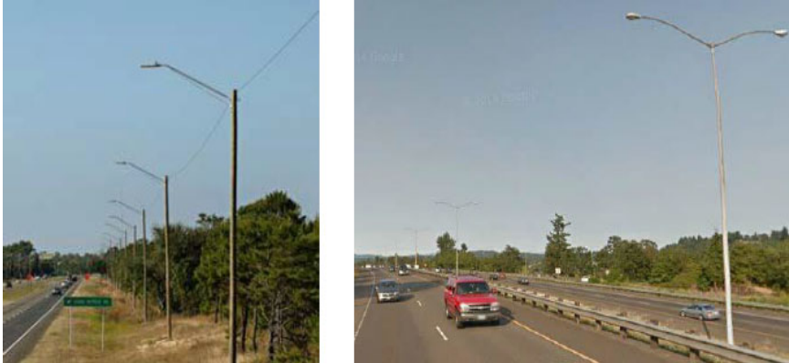
Figure 3-30. Lighting on Roadway Segment
