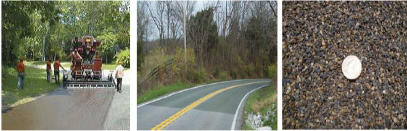
Figure 6-4. High Friction Surface Treatment for Roadway Segment
