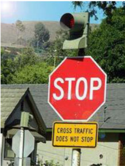
Figure 4-25. Red Flashing Beacon at Minor-road Stop-controlled Intersection
