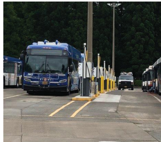
Electric TriMet bus charging at a Portland Metro area charging station.
