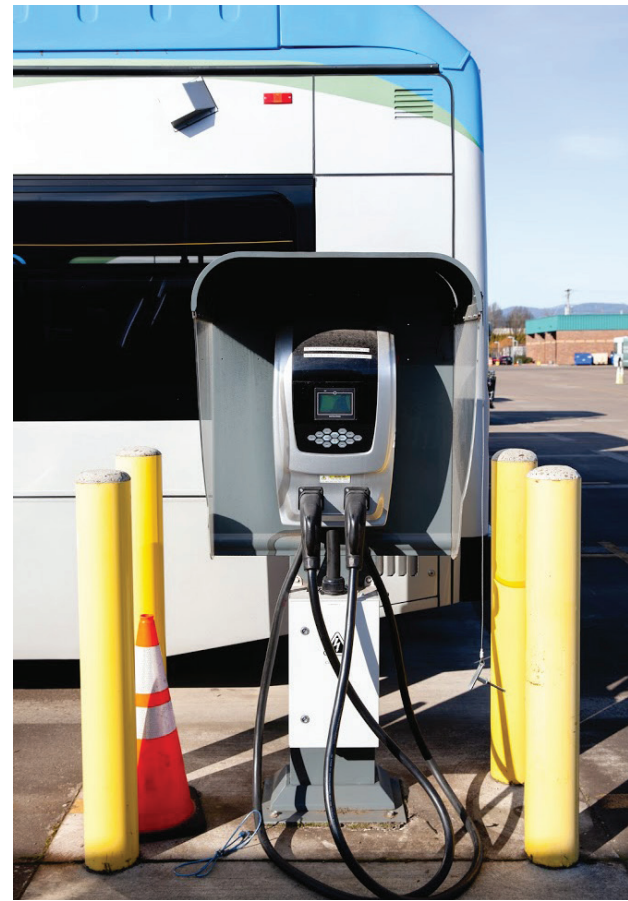
Electric transit bus charging station.
