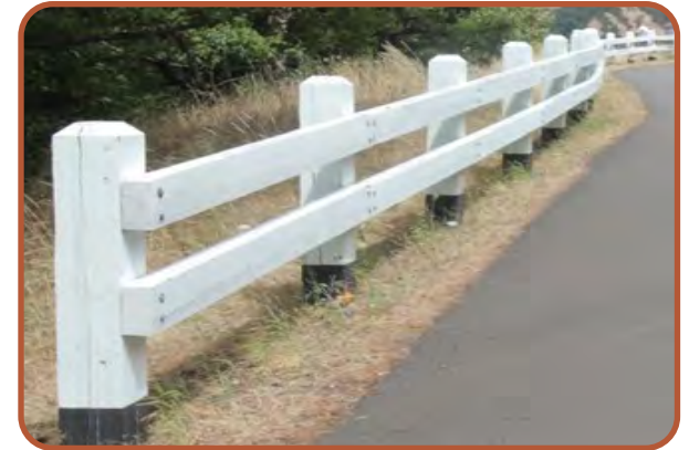
EXHIBIT 9: Recommended white wood railing design. Existing white wood railing at Mitchell Point Trailhead.
