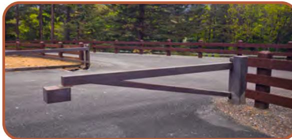
EXHIBIT 17: Recommended simple closure gate design. Existing simple closure gate at Viento Trailhead.
