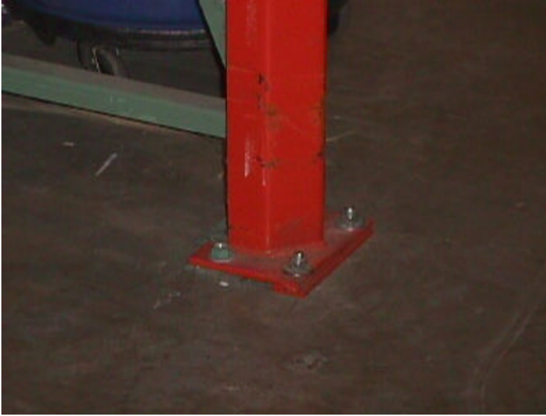
Figure 4. Racks bolted to the floor at the Oregon Lottery warehouse.
