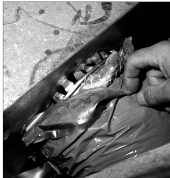
Supply Leak at Take-Off Connection
