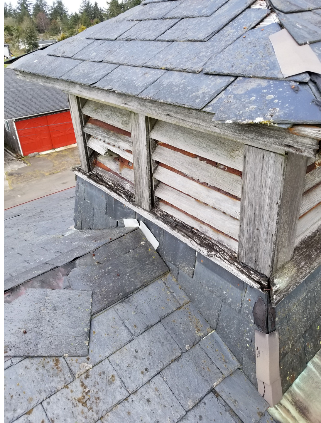
North Cupola before it was destroyed in a storm. Roof Slate in poor condition.
