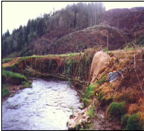
Willow wall construction helped to shade the stream and lower the water temperature. (Photo taken in 1997.)
