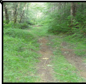
Weyerhaeuser road decommission to help prevent long term culvert failure and road washout.
