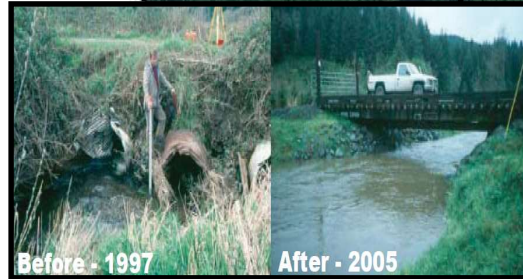
Blocked culverts replaced with a railcar bridge to allow water to flow freely.
