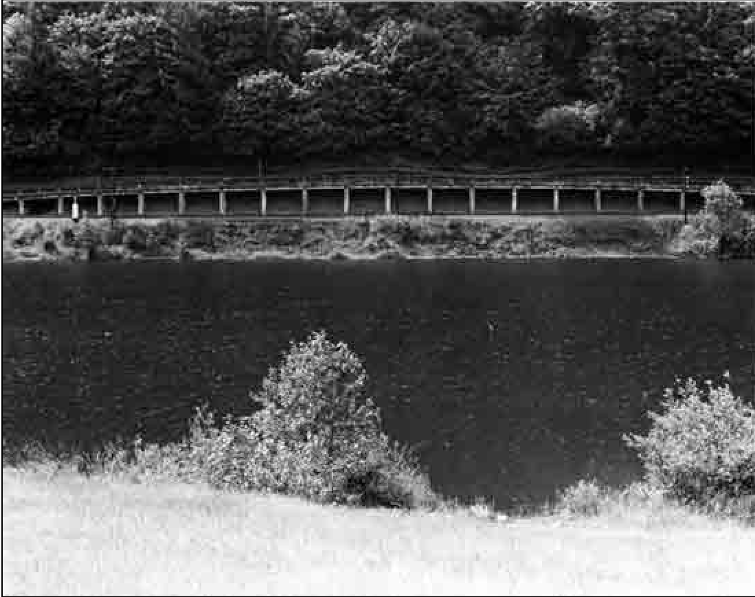
Structure Number 840 Constructed – 1914 Crown Point Highway 125, M.P. 19.50 Reinforced Concrete Slab Multnomah Falls vicinity, Multnomah County Ownership – State of Oregon
