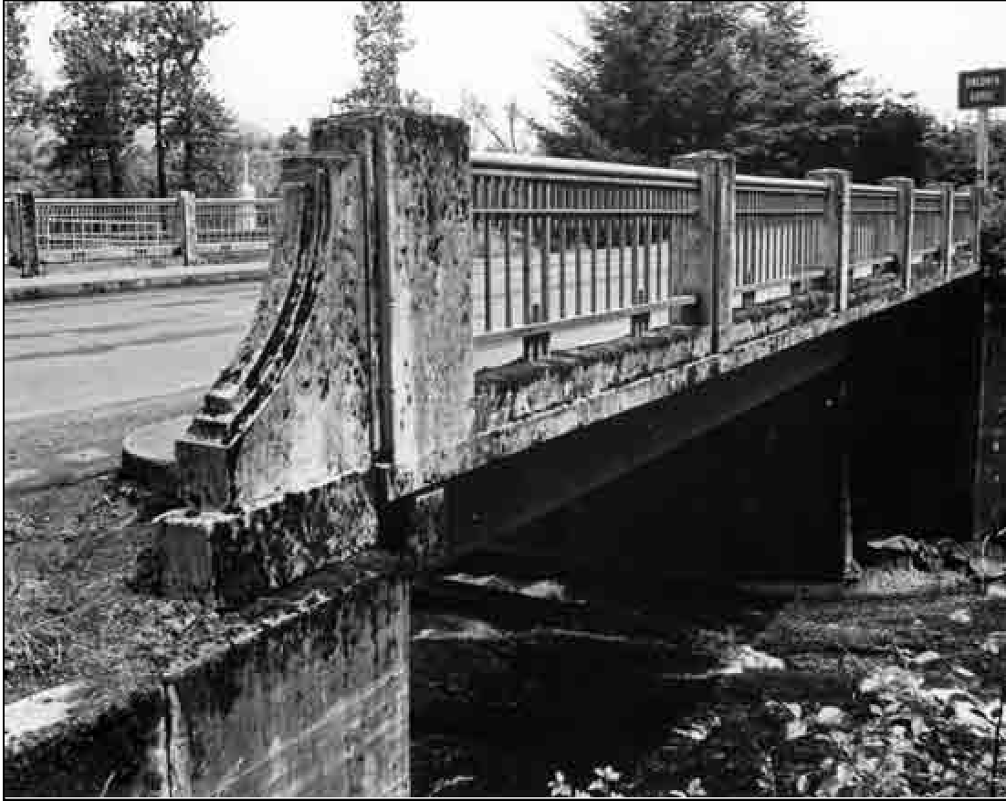
Structure Number 7108A Constructed – 1948 Crown Point Highway 125, M.P. 21.93 Reinforced Concrete Deck Girder Oneonta, Multnomah County Ownership – State of Oregon
