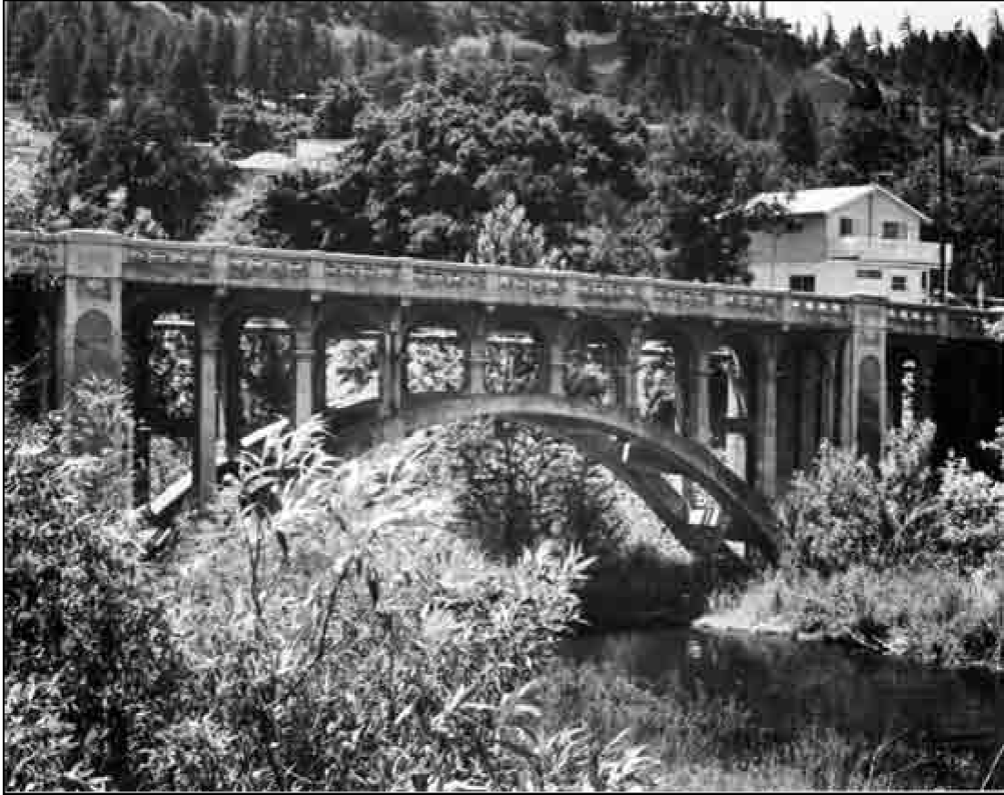
Structure Number 498 Constructed – 1920 Mosier-The Dalles Highway 292, M.P. 0.64 Reinforced Concrete Deck Arch Mosier, Wasco County Ownership – State of Oregon
