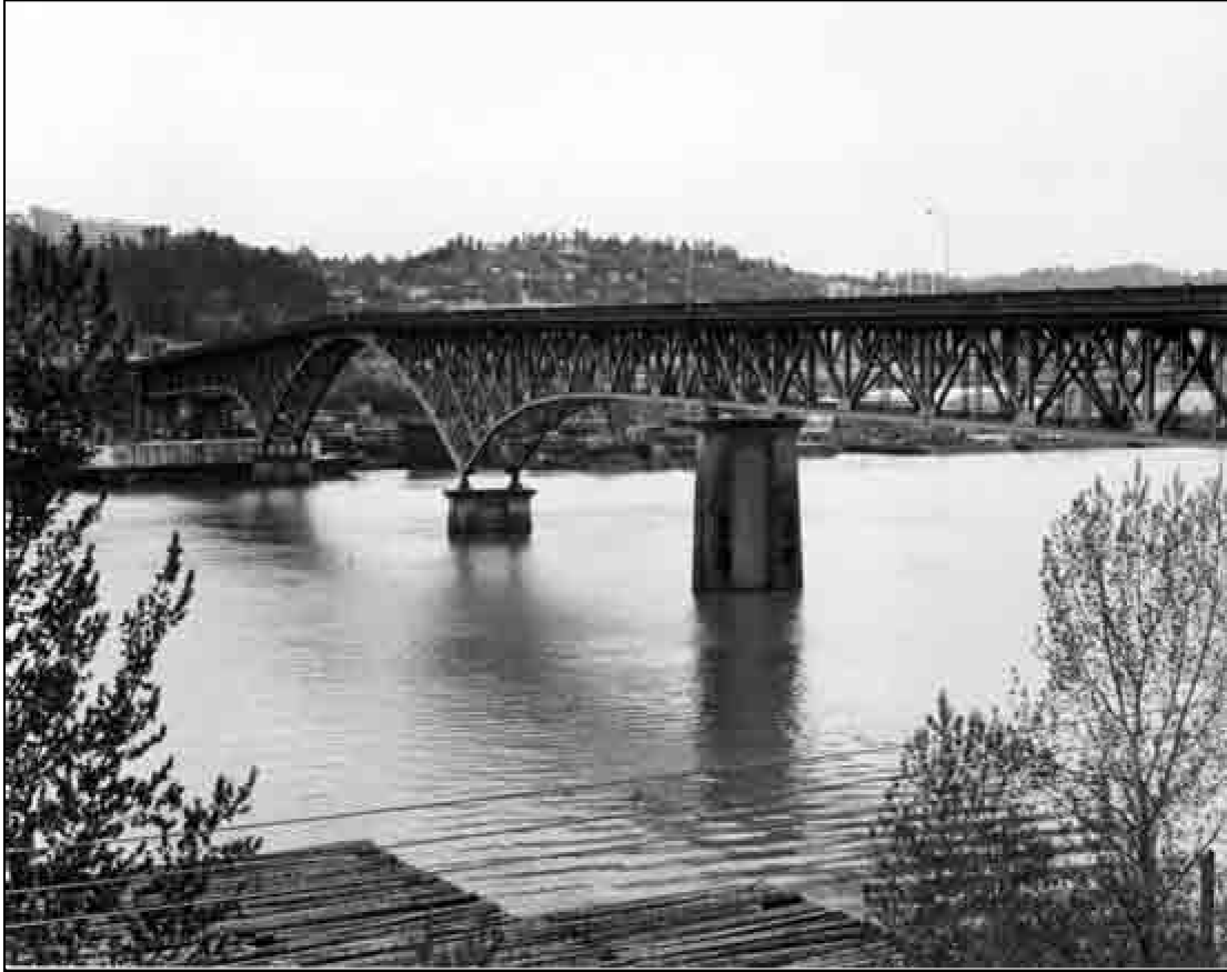
Structure Number 5054 Constructed – 1926 Mt. Hood Highway 26, M.P. 0.77 Steel Deck Truss (Cantilever) Portland, Multnomah County Ownership – State of Oregon
