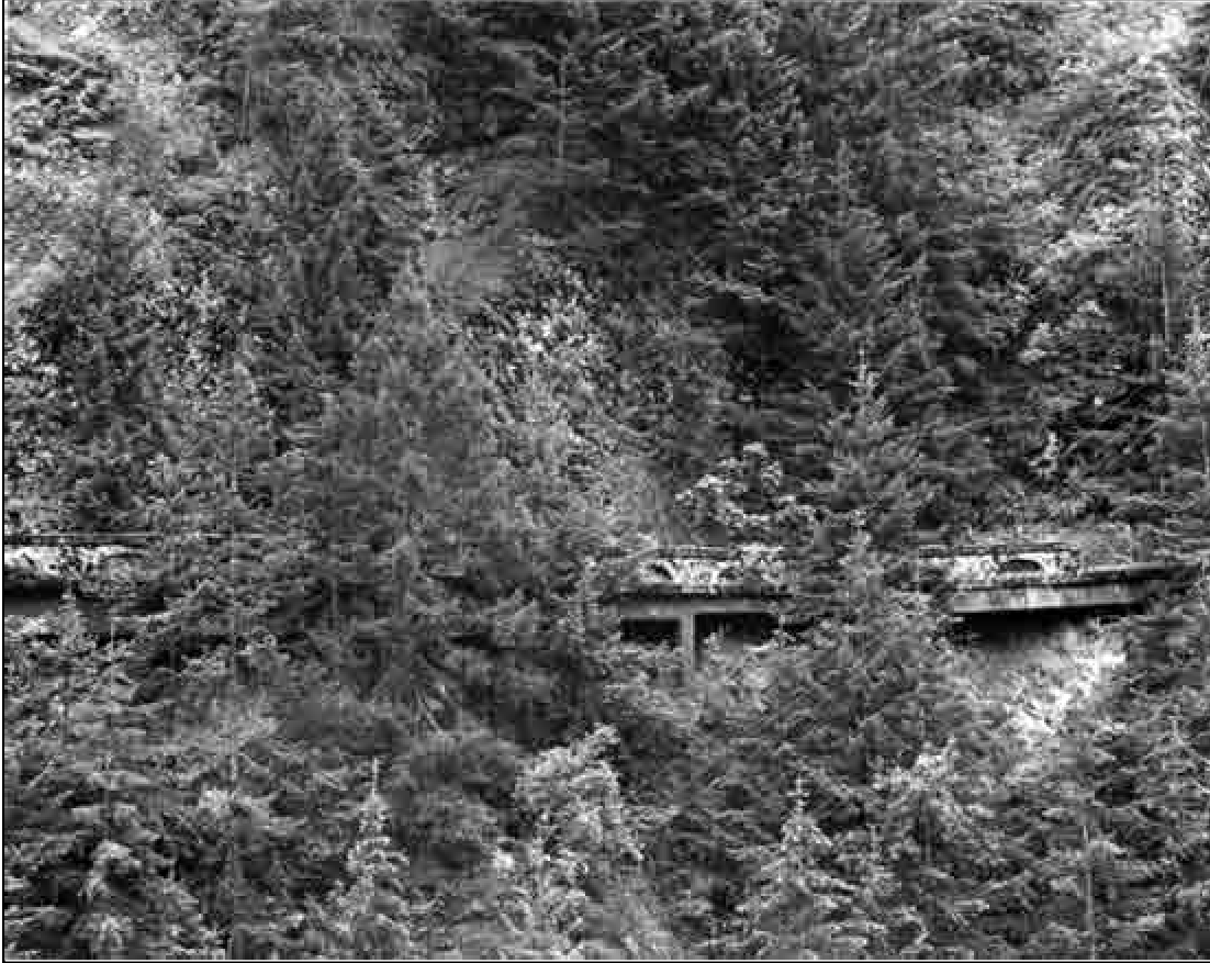
Structure Numbers 17490 and 17492 Columbia River Highway State Trail M.P. 41.25 (Bypassed) Bonneville vicinity, Multnomah County Constructed – 1915 Reinforced Concrete Deck Girder Ownership – State of Oregon
