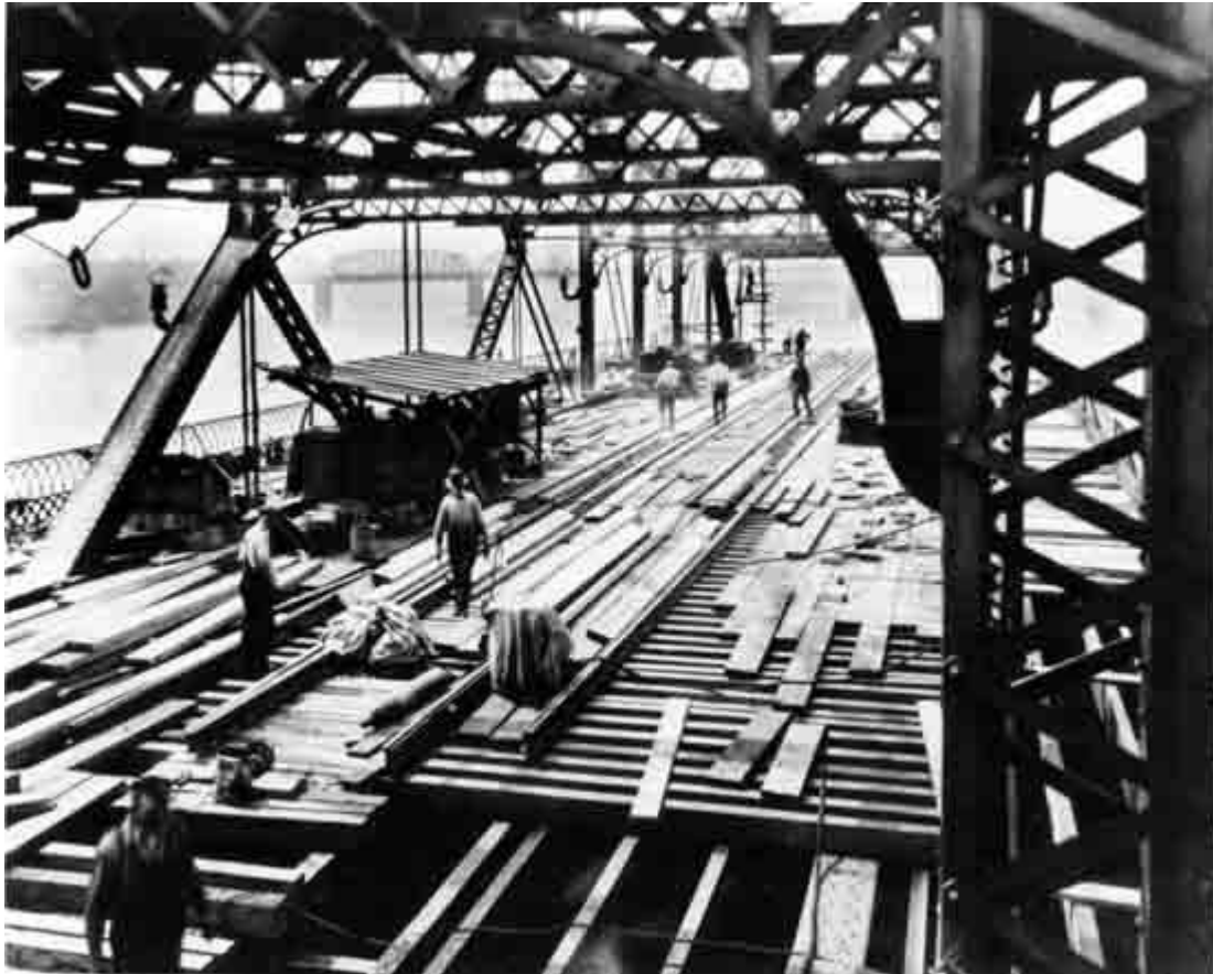
FIGURE 11. The first Morrison Street Bridge, a timber structure built in 1887 across the Willamette River in Portland, was replaced in 1905 by a steel bridge (shown in this 1921 photo). The swing span was open, and deck repairs were underway. The Hawthorne Bridge (1910) appears in the background. A third generation Morrison Street Bridge was completed in 1958.
