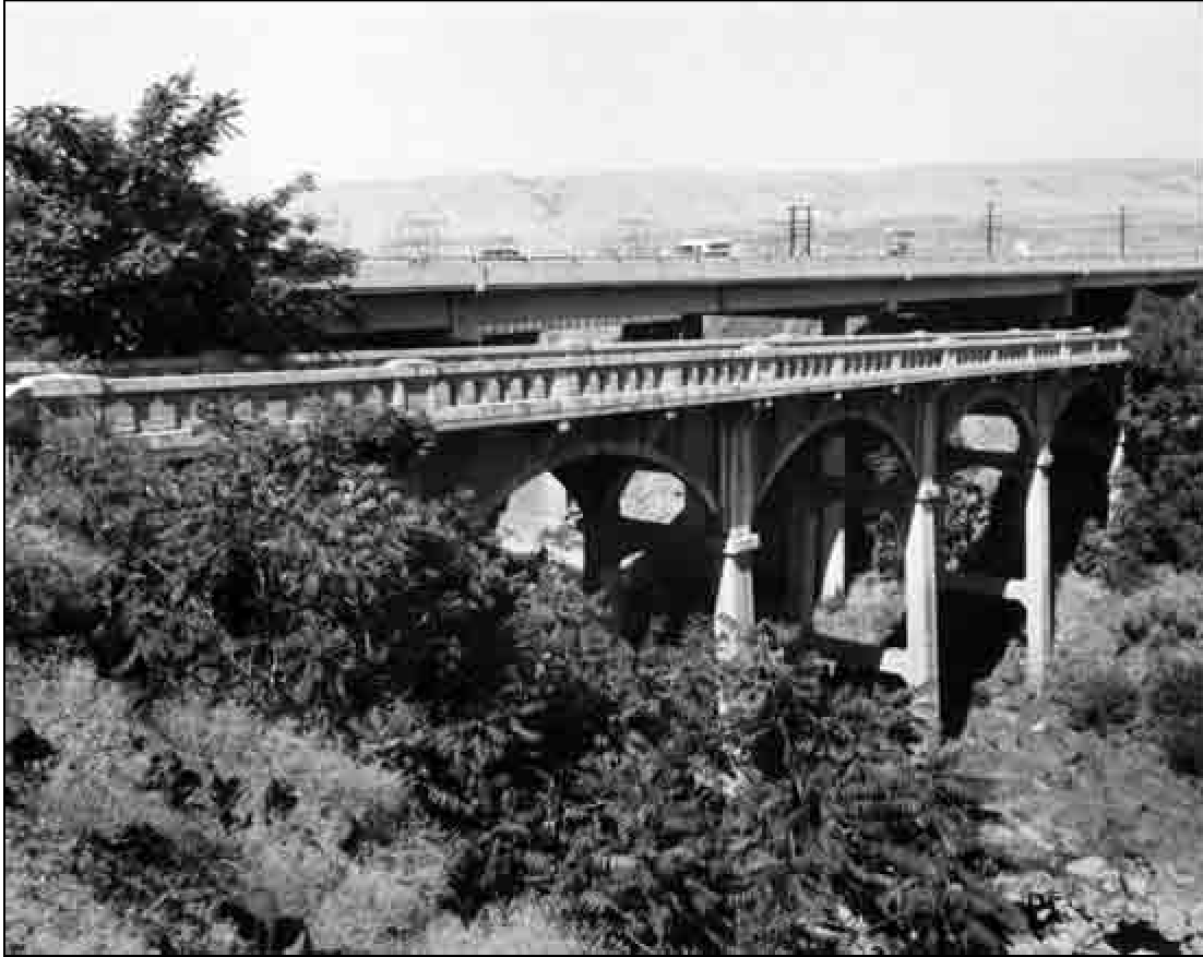
Structure Number 308 Constructed – 1920 State (County) Road Reinforced Concrete Deck Girder The Dalles vicinity, Wasco County Ownership – Wasco County
