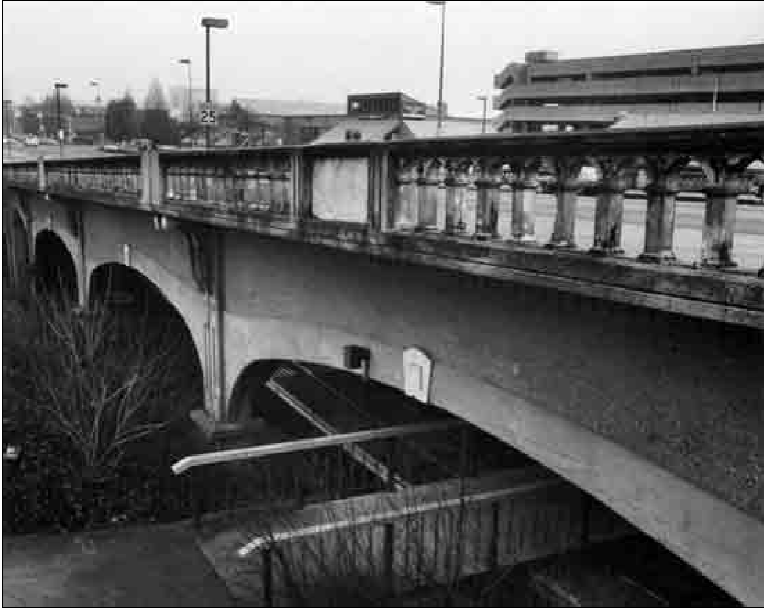
Structure Number 470604 Constructed – 1928 Pacific East Highway 1E, M.P. 50.59 Reinforced Concrete Deck Girder Salem, Marion County Ownership – State of Oregon
