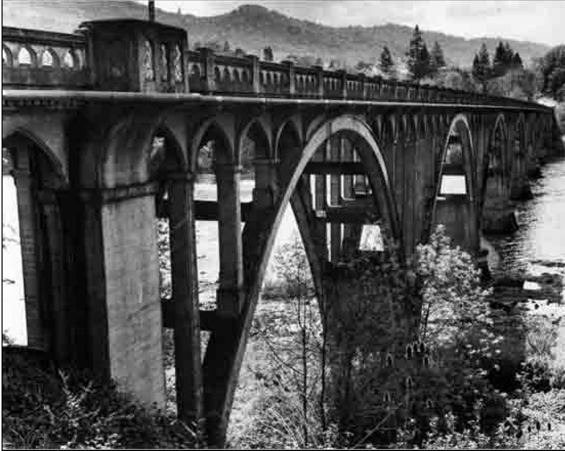
Structure Number 839 Constructed – 1924 Oakland-Shady Highway 234, M.P. 12.21 Reinforced Concrete Deck Arch Winchester, Douglas County Ownership – Douglas County
