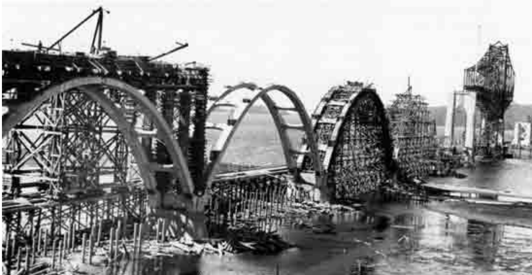
FIGURE 13. The Coos Bay Bridge at North Bend was the longest and most expensive of the five Oregon Coast bridges completed in 1936. (This view is during construction in 1935.) The Coos Bay Bridge was dedicated posthumously in 1947 to Conde B. McCullough, Oregon's early outstanding state bridge engineer.
