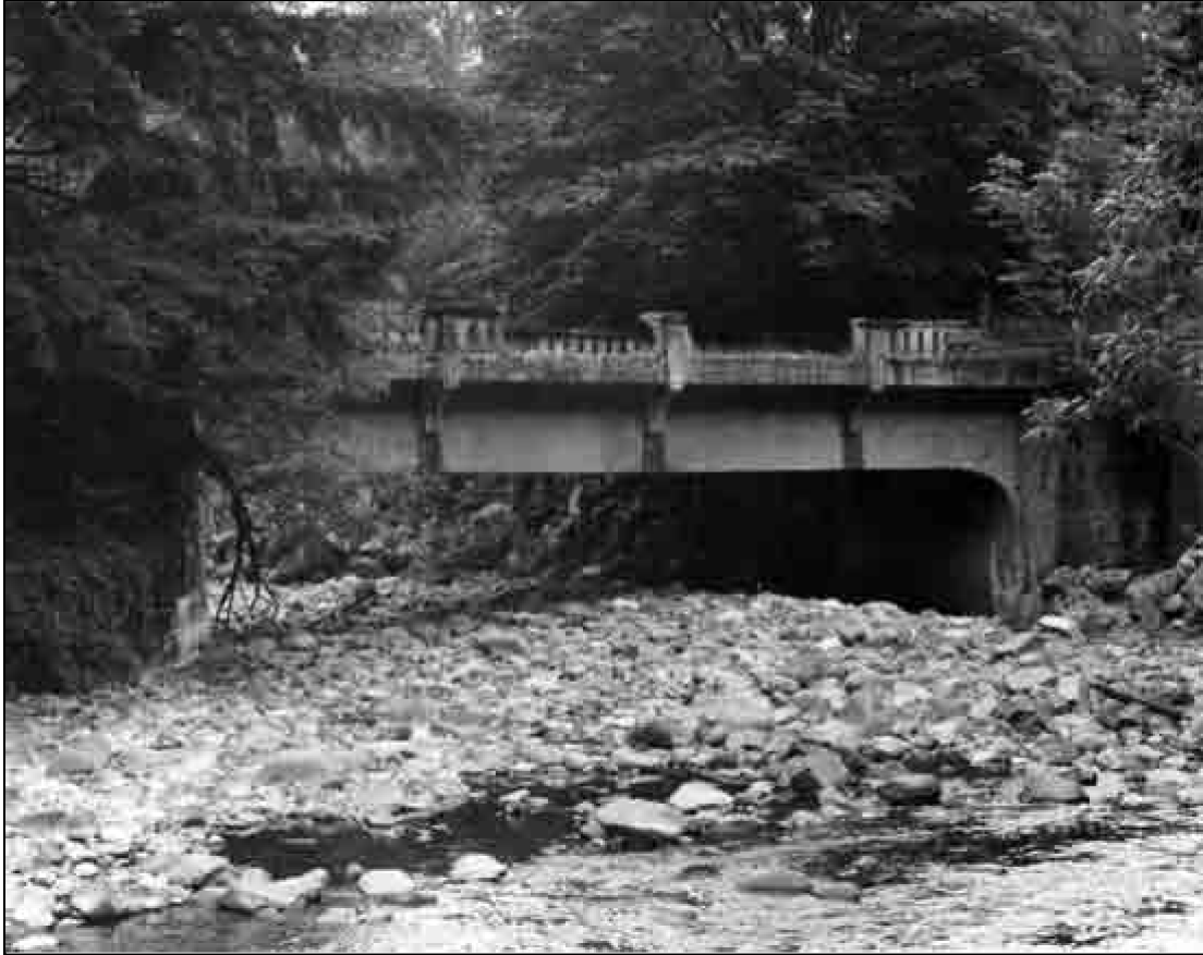
Structure Number 2062 Constructed – 1915 Columbia River Highway State Trail Reinforced Concrete Deck Girder M.P. 40.27 (Bypassed) Ownership – State of Oregon Bonneville vicinity, Multnomah County (Fish and Wildlife Commission)
