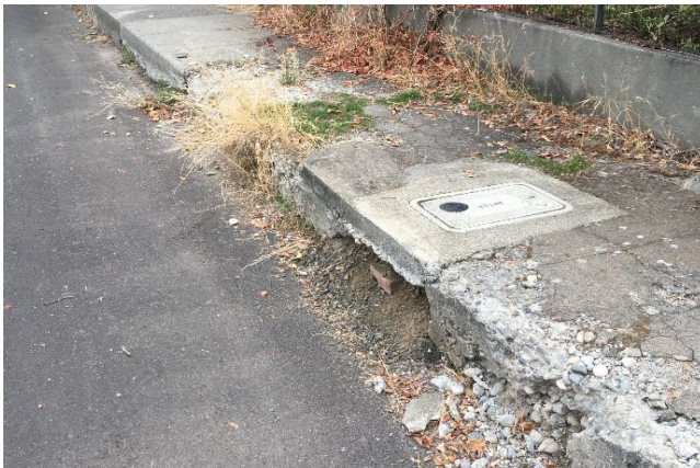
Example - Sidewalk in Need of Improvement
