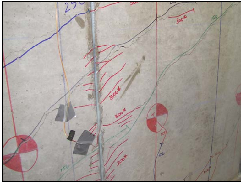
Figure 5.103: B.IT.NC.NS restraint of cracks under load
