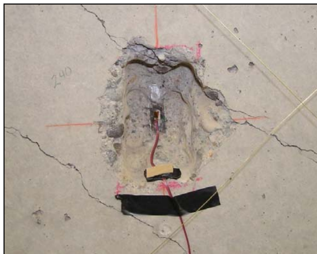
Figure 5.25: Exposure of integrally cast stirrup leg to replace failed strain gage
