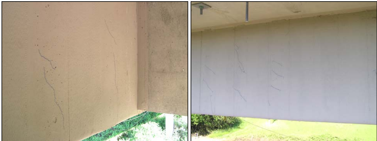
Figure 3.15: Example diagonal cracks observed
