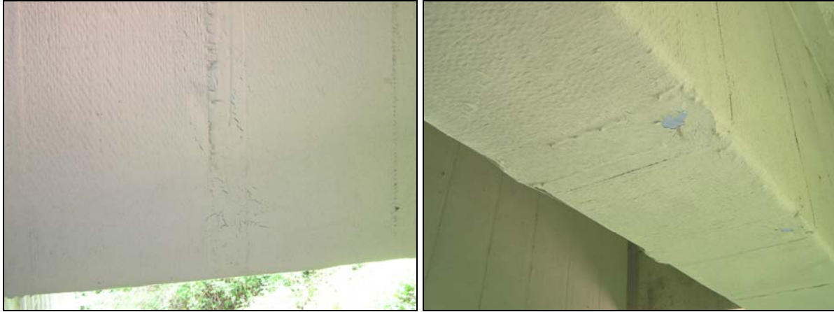
Figure 3.16: Example loss of surface protective coating
