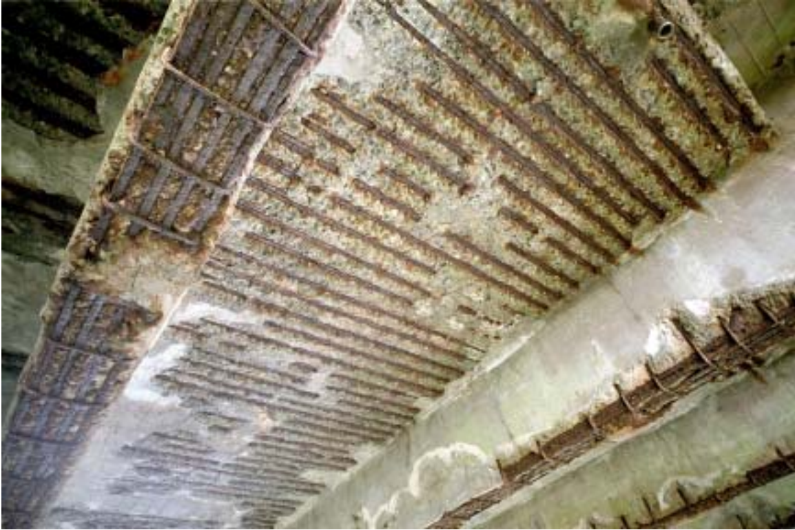
Figure 1.1: Concrete spalling from deck underside at the Big Creek Bridge prior to restoration
