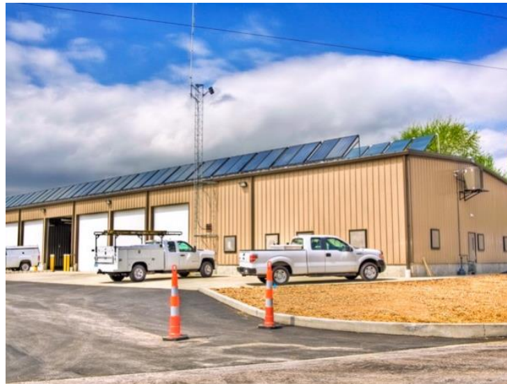
Figure 2.6. Solar air heating system installed on the roof of the maintenance facility in St. Clair, MO (J. E. Foster, 2015).
