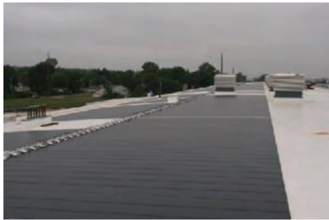
Figure 2.5. Thin-film PV system on a maintenance station roof in South Bend, IN (Lorand et al., 2013).
