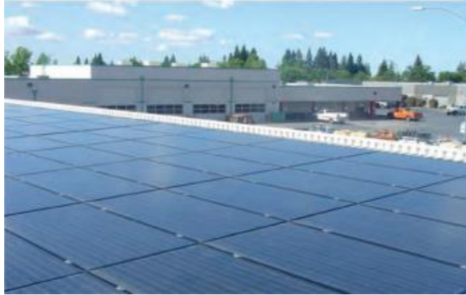
Figure 2.3. PV system at sunrise maintenance station in California (Lorand et al., 2013)
