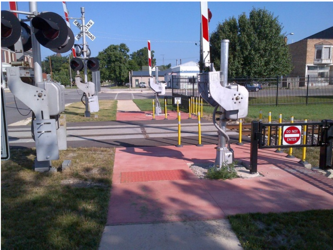
Figure 5.9: Pedestrian Automatic Gates (N/A, N/A, n.d.)
