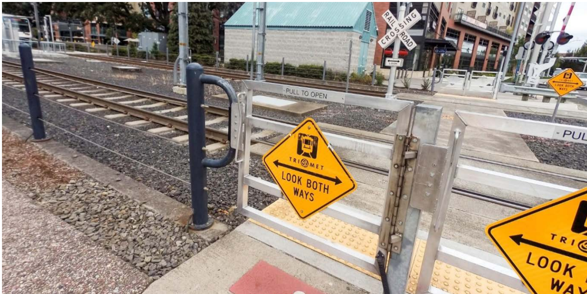
Figure 3.14: Passive gates close off both sides of the crossing closets to the light rail
