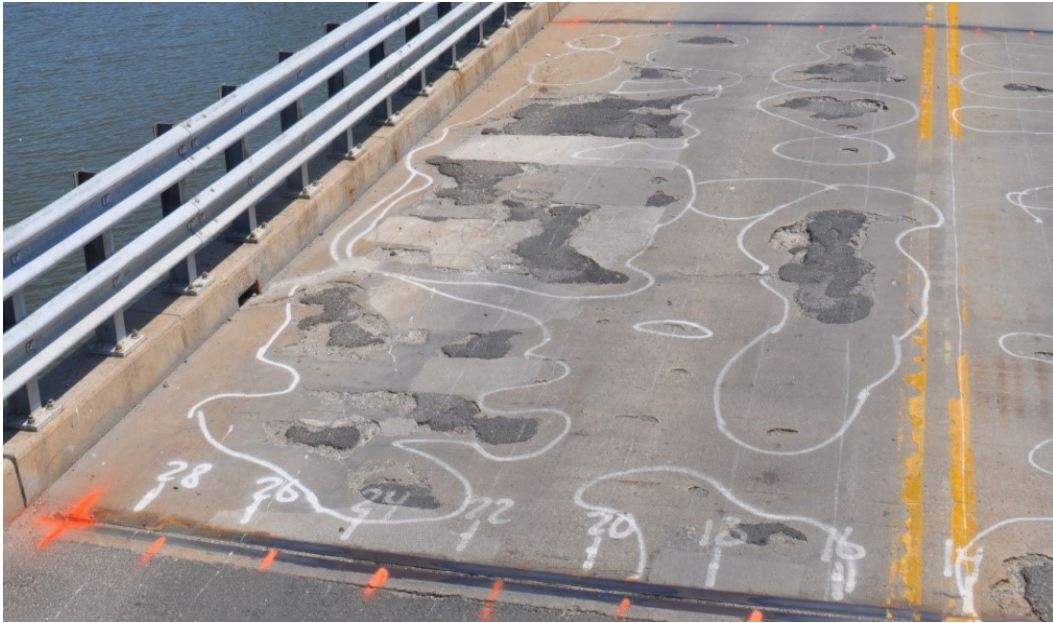
Figure 2.1: Photo of deteriorated bridge deck in Branchport, NJ. Photo courtesy of Thomas Schumacher.
