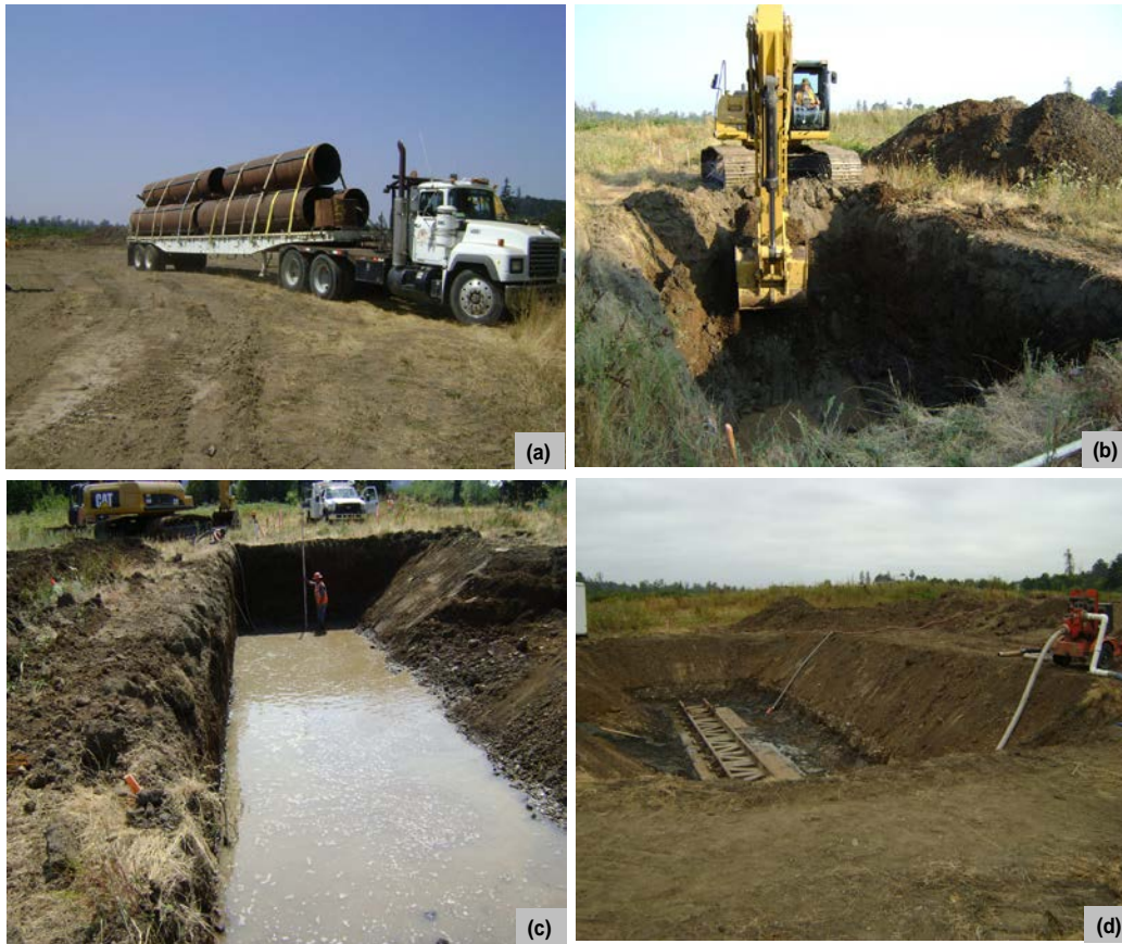
Figure 3.28: Photos showing site preparation activities for the field experiment: (a) transportation of the instrumented pipe the experiment site, (b) excavation of the insertion pit, (c) dewatering the insertion pit, and (d) steel tracks on the leveled gravel bed and steel sheets.
