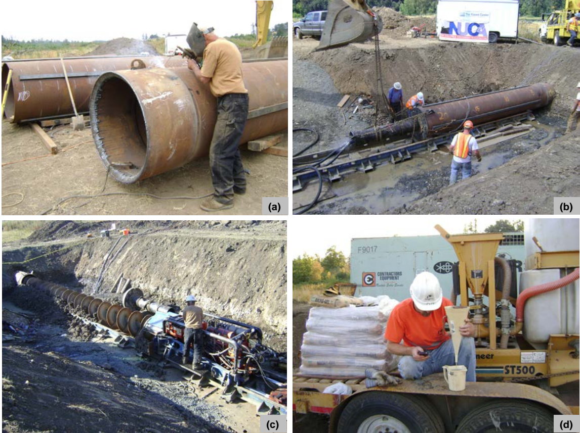
Figure 3.29: Photographs showing experiment activities: (a) welding of the T1 steel cutting shoe to the first pipe segment, (b) pipe ramming in progress, (c) spoil removal using auger boring, and (d) bentonite mixing and field testing of viscosity.
