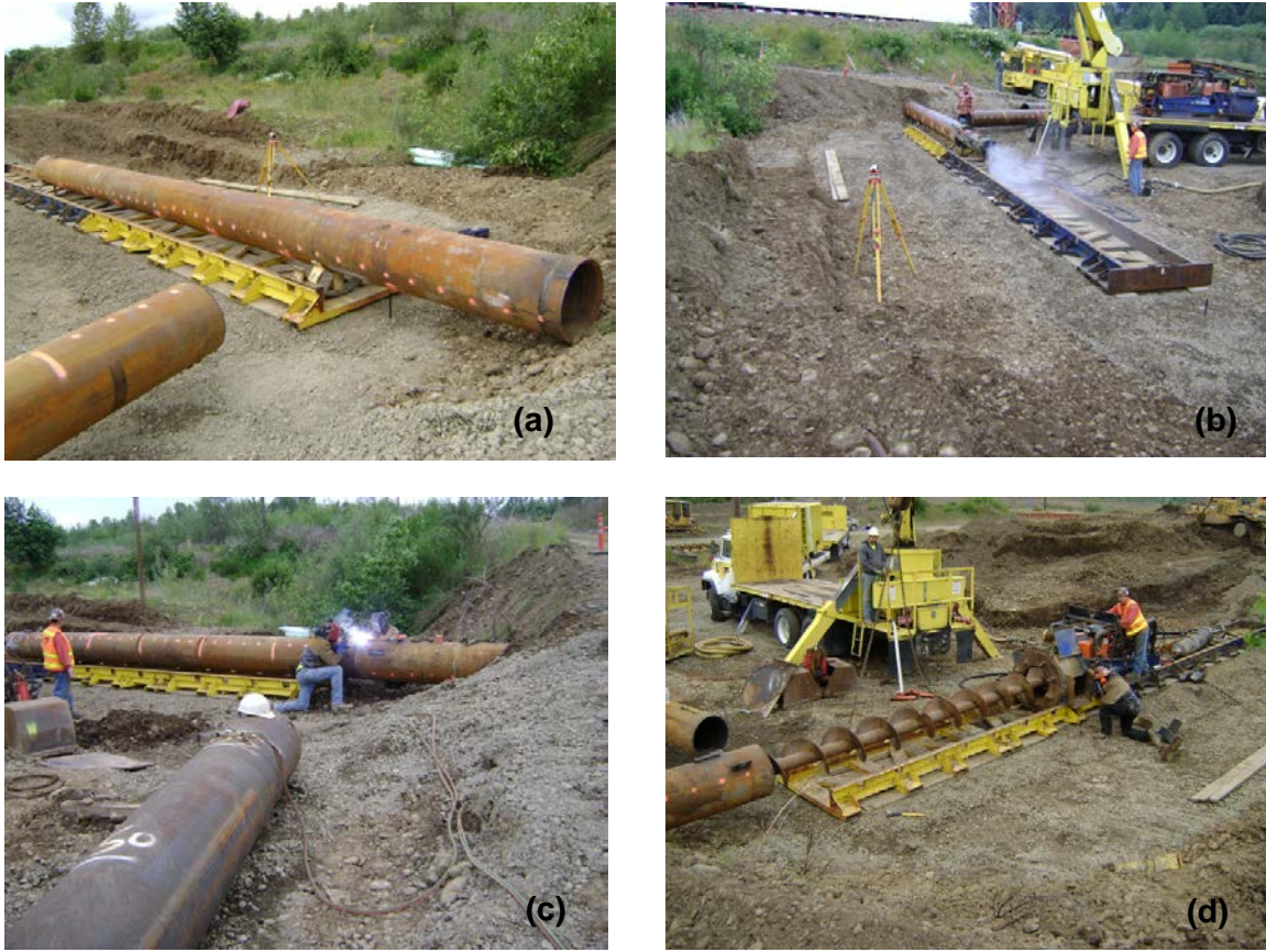
Figure 3.2: Photographs showing construction activities for the Case 1 pipe ramming project: (a) the first segment of the pipe with cutting shoe welded at the leading edge and situated steel auger boring tracks, (b) the ramming process under the embankment, (c) welding the second segment of the pipe, and (d) spoil removal using auger boring.
