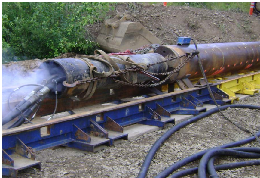
Figure 2.6: Photograph of 400 mm pneumatic hammer driving 600 mm diameter pipe pipe (corresponding to Case 1, described in Chapter 3).
