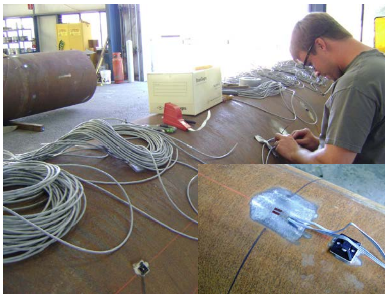
Figure 3.27: Pipe instrumentation with strain gages; note, pairs of gages were installed to provide redundancy.
