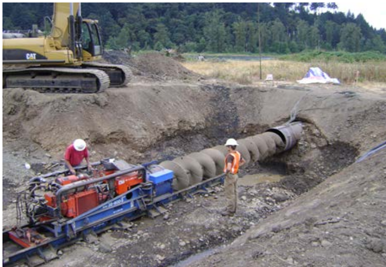
Figure 2.9: Auger boring machine removing spoil from 1060 mm pipe (corresponding to Case 6, described in Chapter 3).
