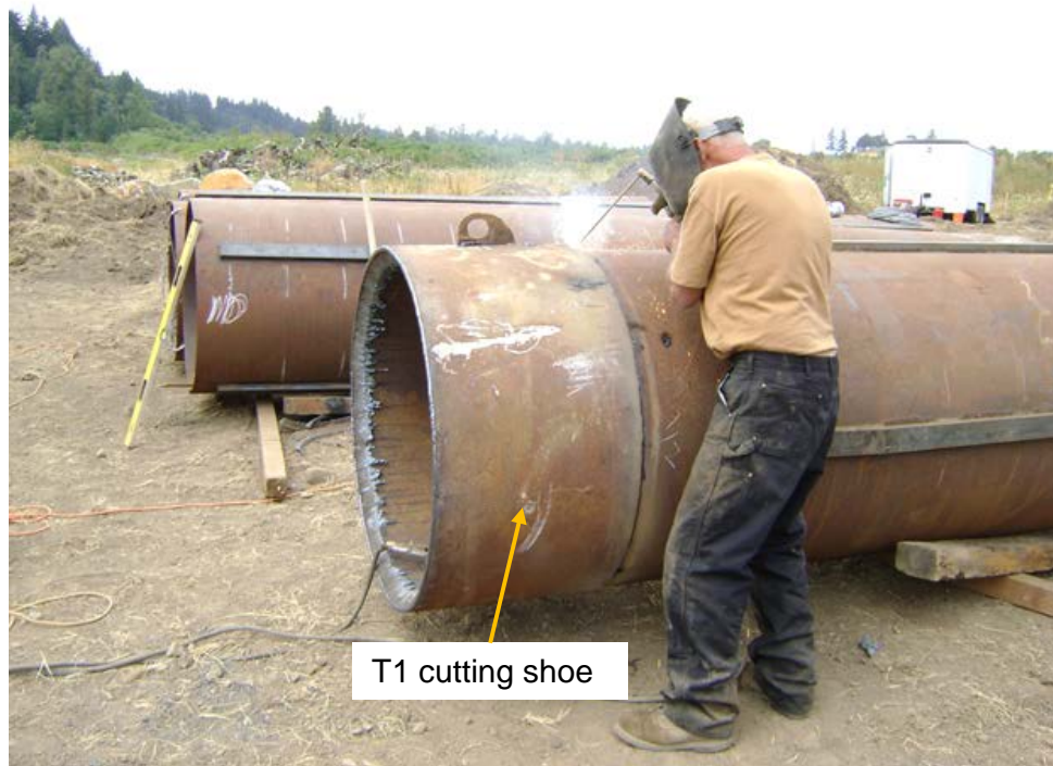
Figure 2.8: T1 cutting shoe being welded to 1060 mm diameter pipe pipe (corresponding to Case 6, described in Chapter 3).
