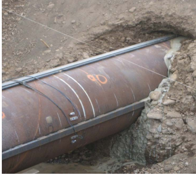
Figure 6.11: Photo showing the bleeding loss of the lubricant due to the likely damage of the lubricant hose close to the insertion of the pipe.
