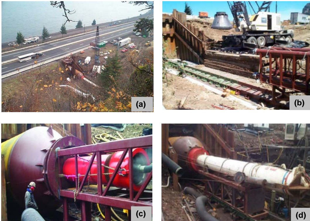
Figure 3.11 Photos showing activities related to Perham Creek culvert replacement project: (a) pipe ramming operation under Interstate 84, (b) launch pit set-up, (c) 800 mm pneumatic Grundoram Apollo hammer ( J.W. Fowler, personal communication, 2012 ), and (d) 915 mm hydraulic IHC S-280 hammer ( ODOT 2010 ).
