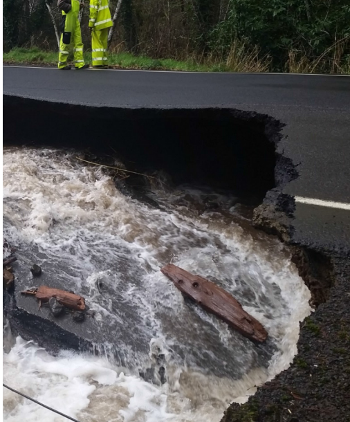
When culverts failed, inundation and debris did significant damage to county roads. Credit: Tillamook County Roads
