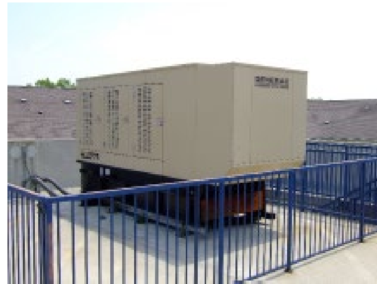
Creswell Airport (Hobby Field) 2020 – Emergency Stand-by Generator
