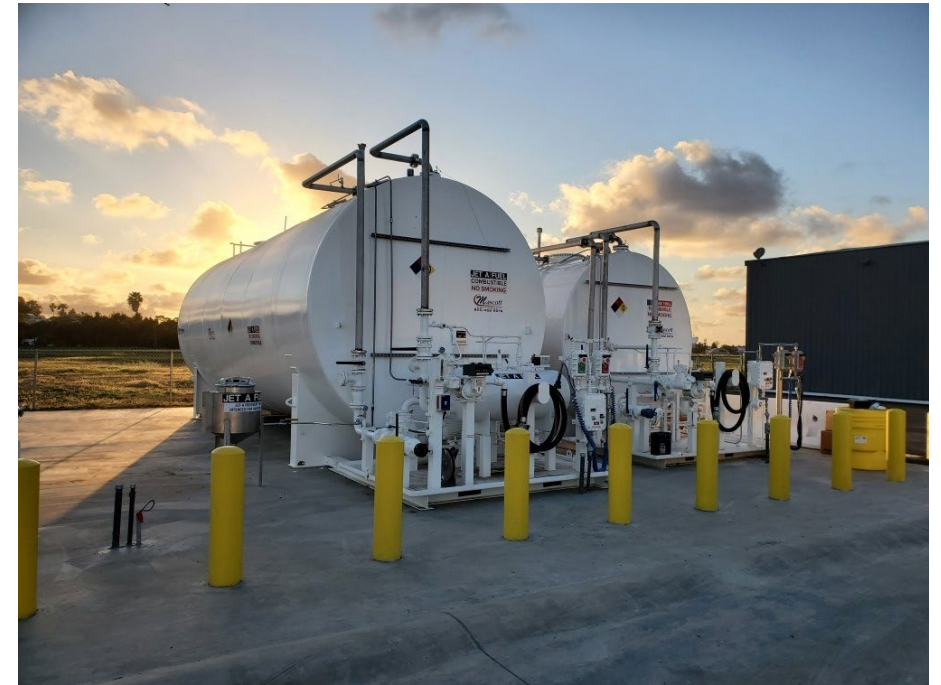
Example of fueling equipment
