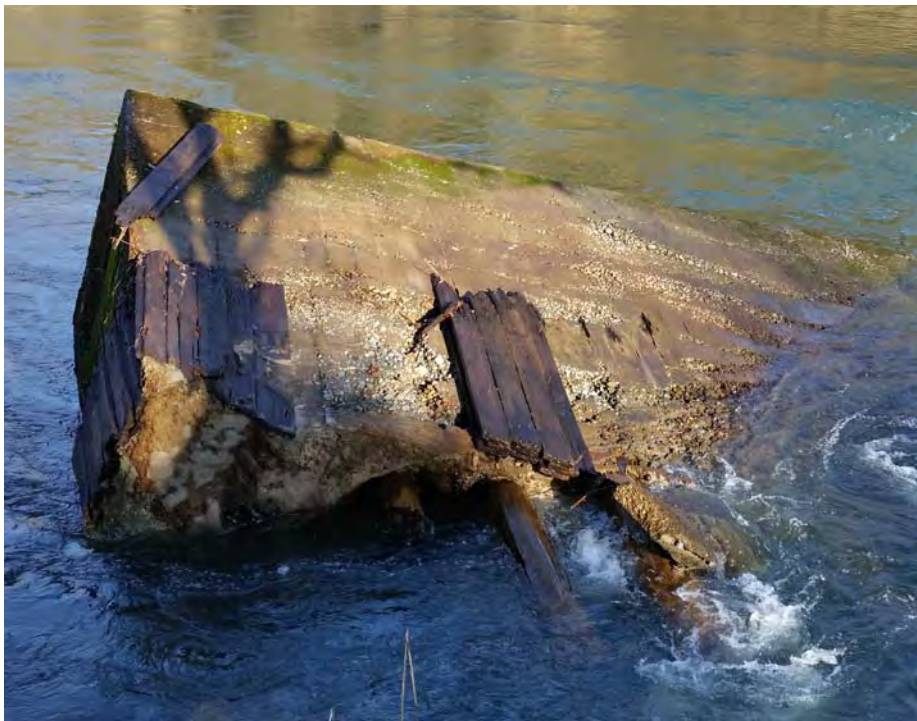
View of concrete railroad trestle remnant at 17/2634-1 near the south bank of the Molalla River. The view is towards the north.
