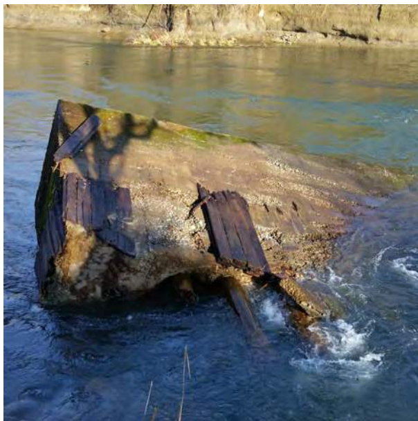
Photo 11. Concrete and wood remnant of the former Willamette Valley Southern Railway trestle crossing the Molalla River (site 17/2634-1). The view is towards the north.
