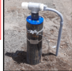
COAR 2021 Cycle project already done! Beaver Marsh's First COAR grant - new well head completed. Great job!
