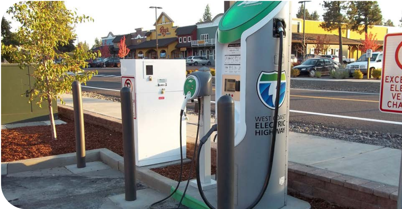
| Electric vehicle charger installed in a parking lot in Oregon.
