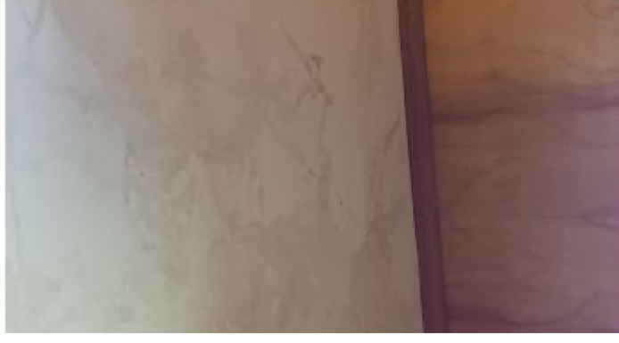
is of the building exterior, water staining on the
