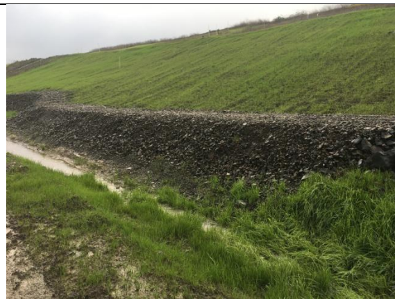
Repair area where outside of north berm had some soil sloughing. This area is in good condition.
