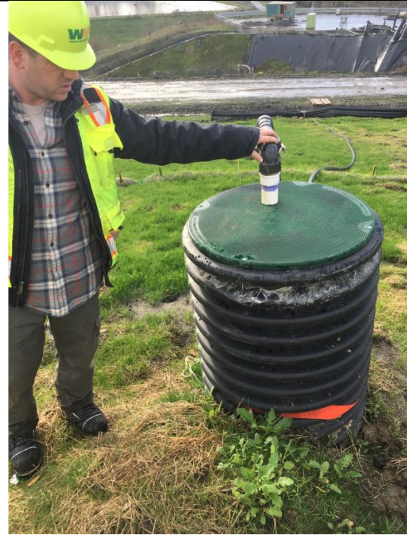
Access point for French drain, one of several installed on the sideslope to address leachate seeps.
