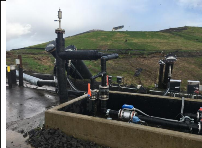
Concrete containment area for controls for Module 9 leachate management system. Previous inspection report noted hose running from the air relief valve (on vertical pipe) to the concrete containment area because leachate was getting into this air line. This problem has been corrected.
