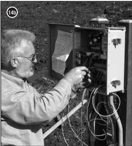
Wire control panel.
