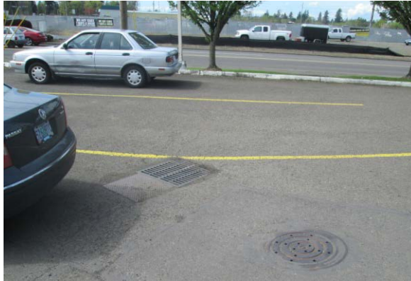
Figure 1: A catch basin (square feature) that collects stormwater from a parking lot and conveys the stormwater to a drywell (circular feature)
