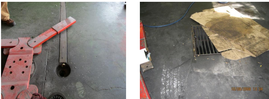
Figure 1. A circular floor drain (left) and catch basin floor drain (right) that drain to a drywell at an automotive-related business. These devices are automotive waste disposal wells.
