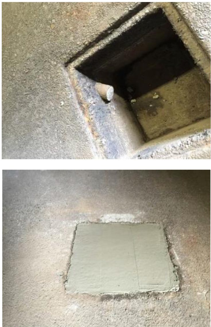
Figure 6. Decommissioning of a catch basin-style floor drain. The top picture shows the floor drain after disassembly and cleaning. The bottom picture shows the floor drain after it has been filled with cement. Note that the piping leading from the catch basin is capped prior to cementing.
