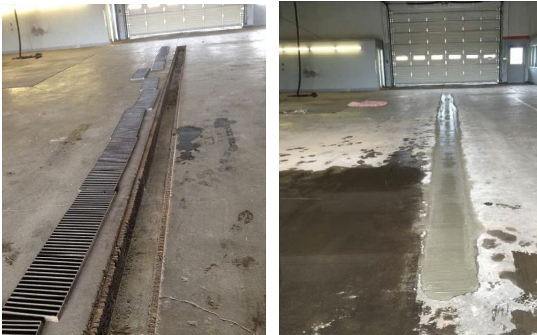
Figure 5. Decommissioning of a trench-style floor drain. The picture on the left shows the floor drain after disassembly and cleaning. The picture on the right shows the floor drain after it has been filled with cement.
