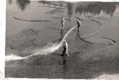
Fred Korki, Art Piddie and Louis Tenny washing down Reservoir #2 floor - side walls have been cleaned and sterilized. May 1959
