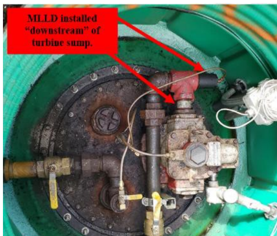
Figure 2.0 - Mechanical Line Leak Detector is installed immediately adjacent to the turbine
