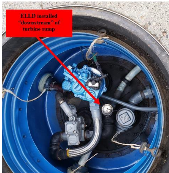
Figure 4.0 - Electronic Line Leak Detector installed off of turbine sees pressure in both directions.
