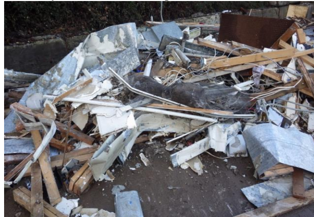
Image 10. Drop box of residential remodeling debris that was tipped and found to contain asbestos-containing thermal system insulation wrap.
