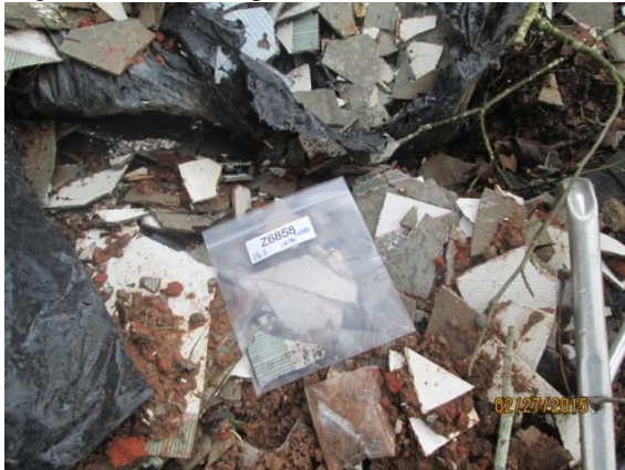
Image 9. Fragmented residential siding containing 30% Chrysotile asbestos CAB panels frequently fragment into friable pieces.
