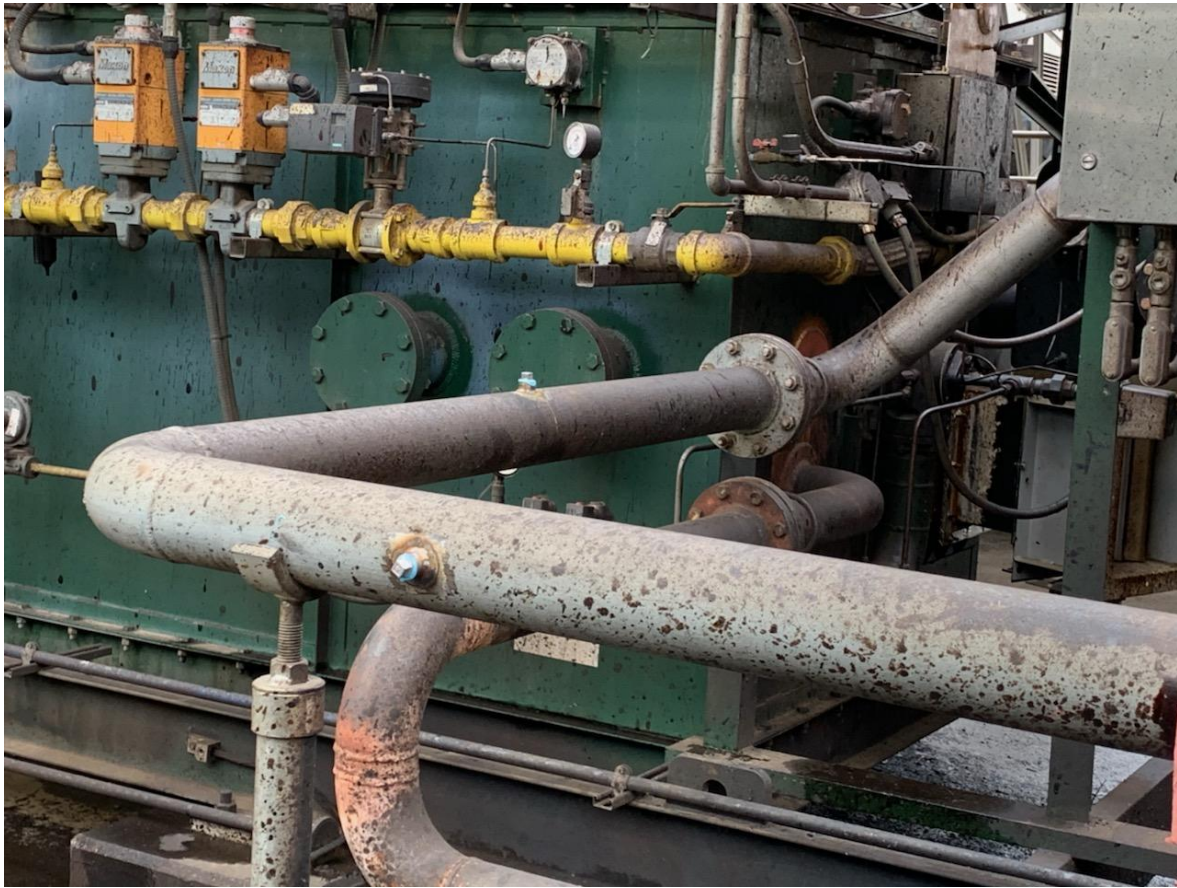
Top Inlet line ~ 6"
