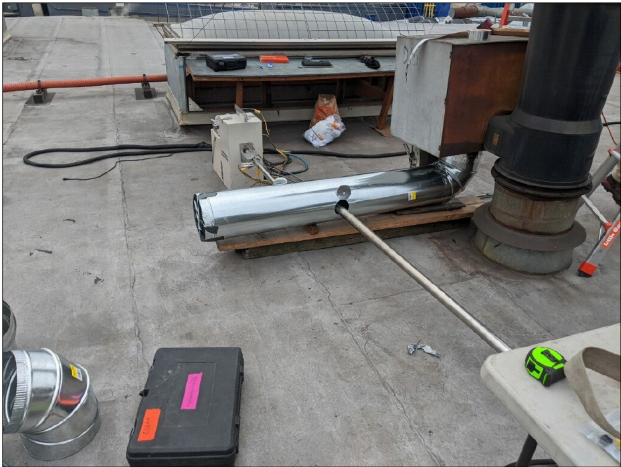
Figure 2. Quick Draft Fan Inlet Duct Photo
