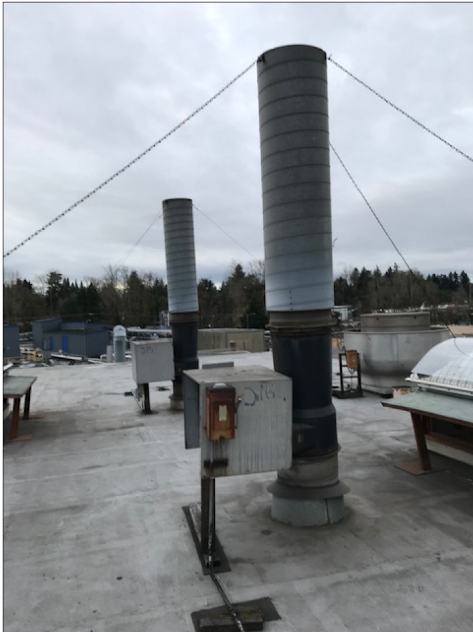
Figure 1. Discharge Stack Photo
