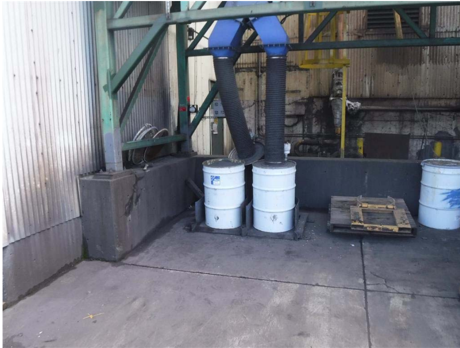
Photo 1: Baghouse 26 collection drum disconnected immediately prior to sampling
