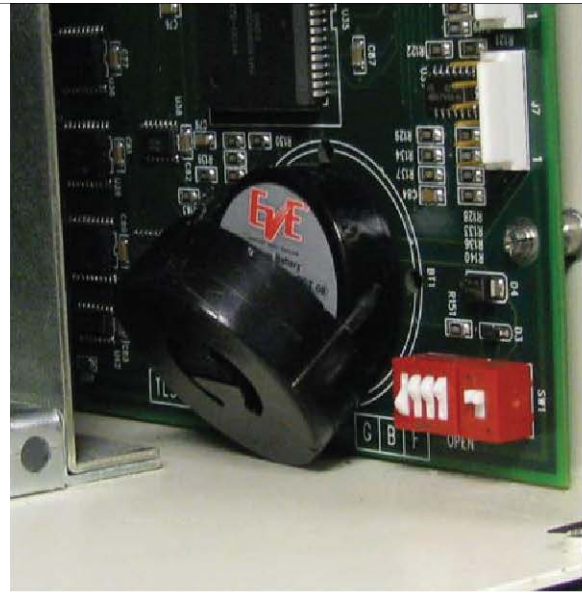
B. Battery Cover Dislodged
