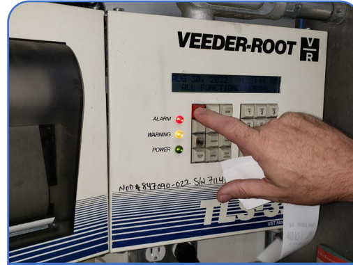
Clear tank gauge alarm
